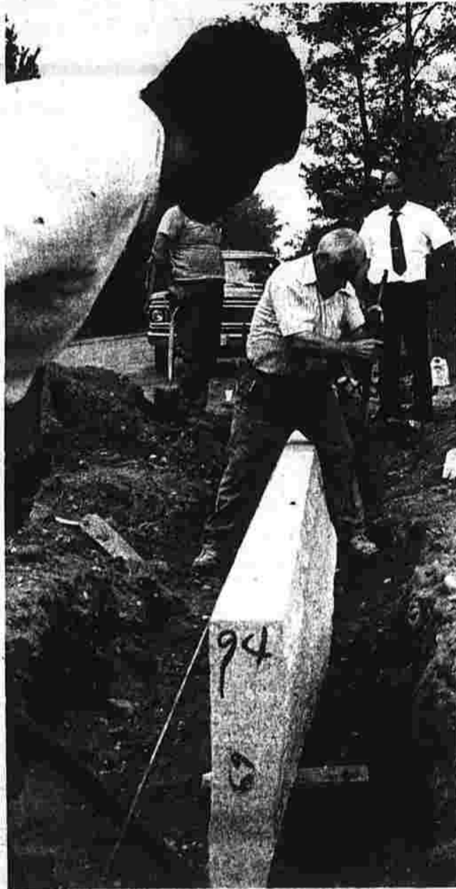
Installing new curbs. Granite curbs were installed on a Thompson Road sidewalk construction Wednesday afternoon. Walter Senkow, town engineer, watches from the rear as Joe Wilkovich adjusts the curbing while John Almeida, front, keeps the curb on line. (Herald photo by Chastain)
